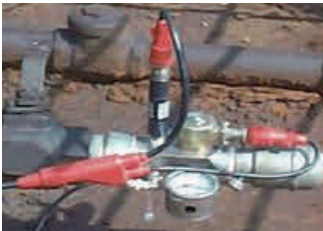
Well Analyzer Gas Gun & PT
